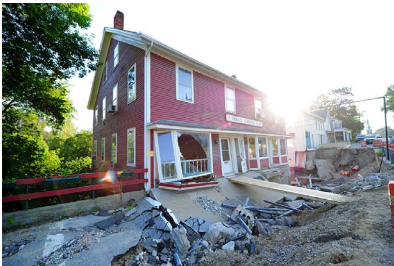
Structural damage in Vermont
